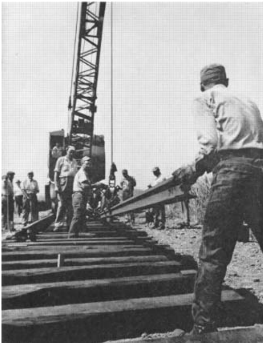
ERIE MEN LAY RAIL through the age-old rushes of the Jersey Marshes toward the new Merchants Refrigerating Co. facility.
