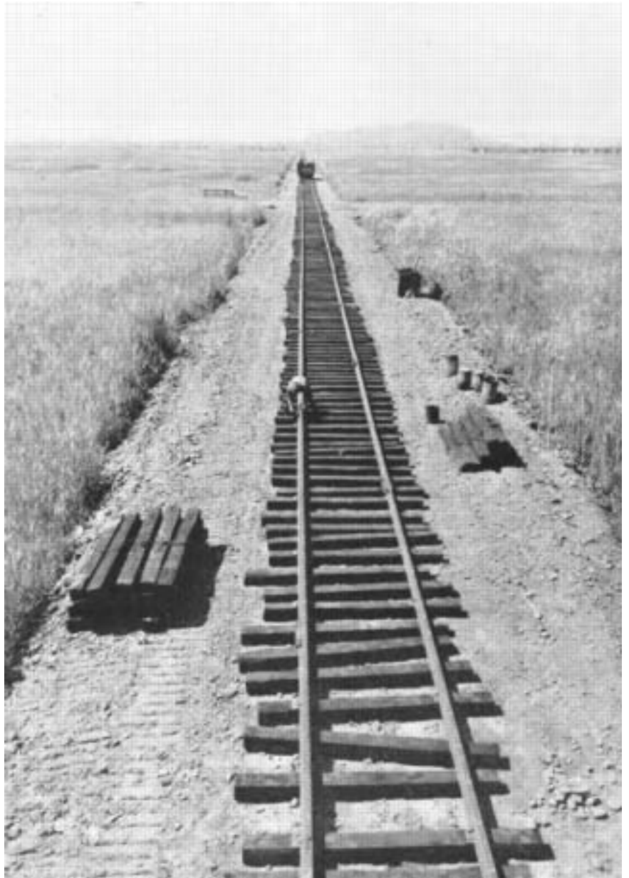
NEW RAIL ROUTE cuts through the unmarked wilderness of the marsh in a straight line.
