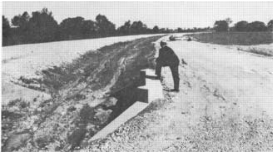
FLAT IS THE WORD for the land around the falls. Here is the new Erie roadbed on the right, close to the point it leaves the present line.
