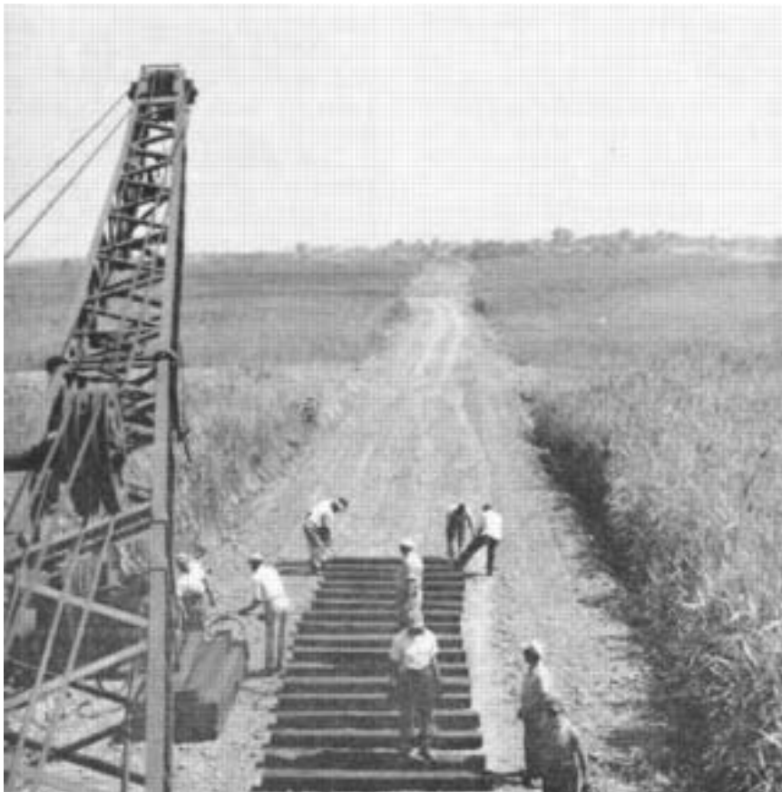
TIES ARE LAID OUT ahead of the rail-laying crane as the new line cuts through the marsh.
