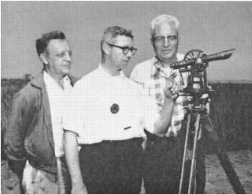
SURVEY PARTY checking alinement of roadbed through the marsh: left to right, Albert T. Decker, inspector, Jersey City; Edward K. Herling, Binghamton and William J. Galloway, resident engineer, Jersey City.
